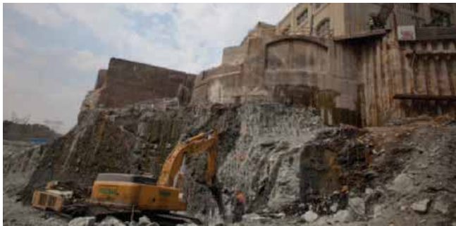
At the $450-million Holtwood hydro expansion project in Lancaster County for Pennsylvania Power & Light, MD&B is working with Walsh Construction, breaking rock to make way for a new powerhouse that will double the capacity of a 1910 plant.
