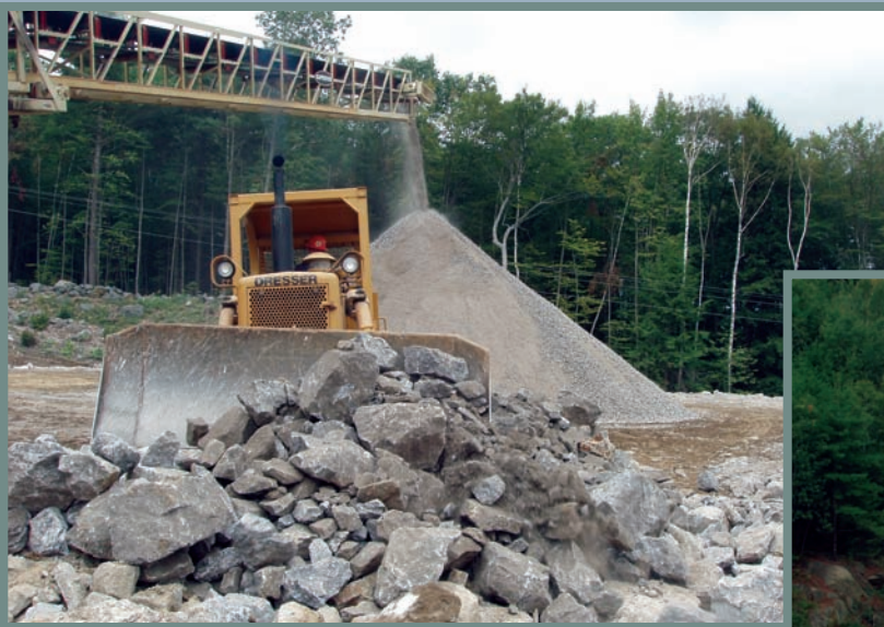
Above: As finished crushed stone is deposited in stockpile in background, a Dresser TD15C dozer spreads blasted rock fill. Right: Rock has been blasted to move wall of ledge back to a safe distance from the southbound barrel of I-89.
