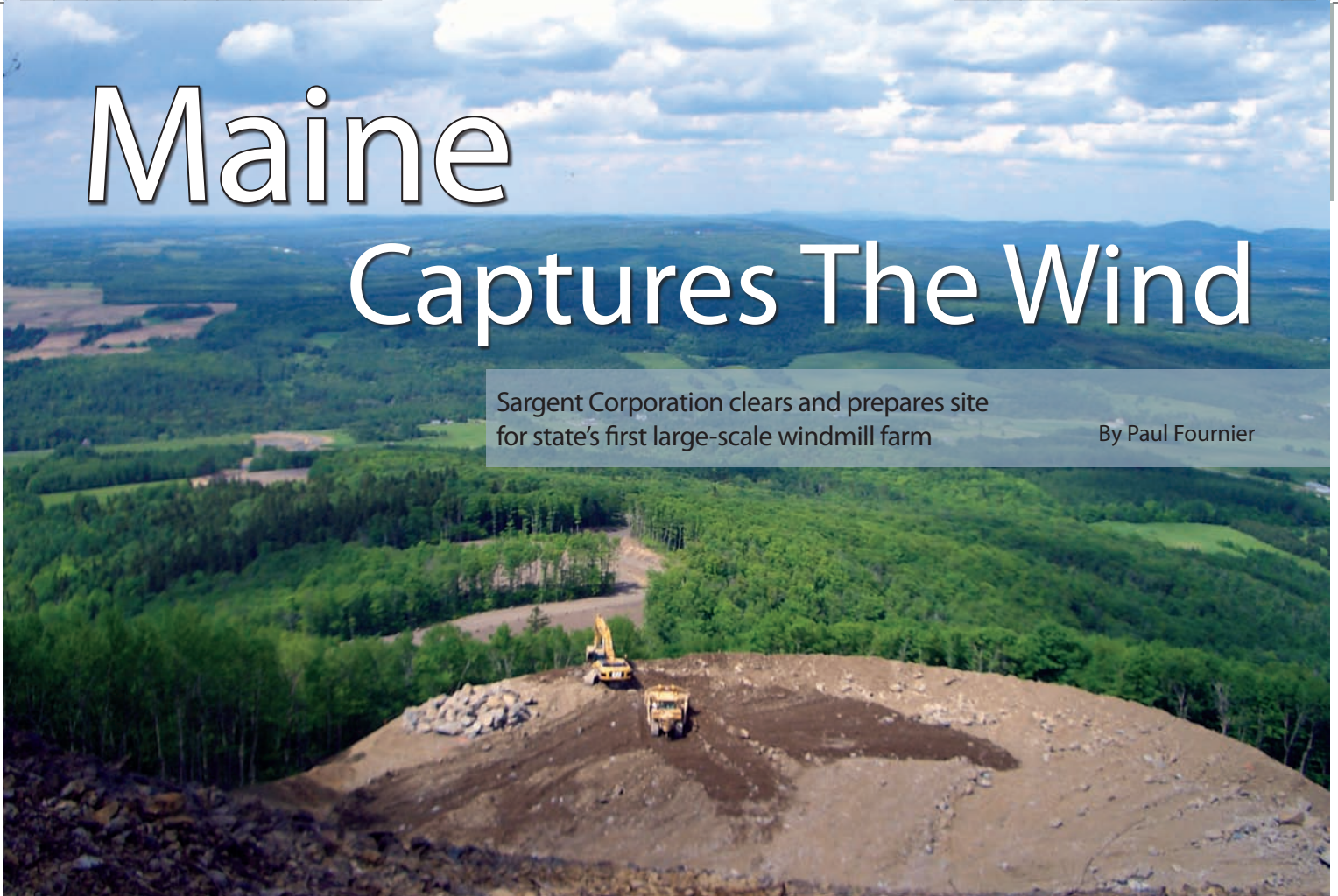
Photo taken from one windmill tower pad of ongoing excavation at a second pad illustrates the difference in elevation of the windmills.
