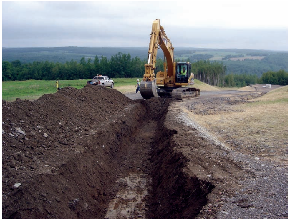
One of Sargent's Cat excavators digs trench for conduit that will carry generated power to utility grid.
