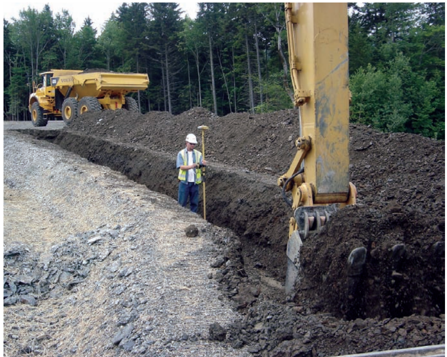
A Sargent Corporation worker uses Topcon HiPer+ survey rover to check grade of utility trench at windmill project in Mars Hill, Maine.
