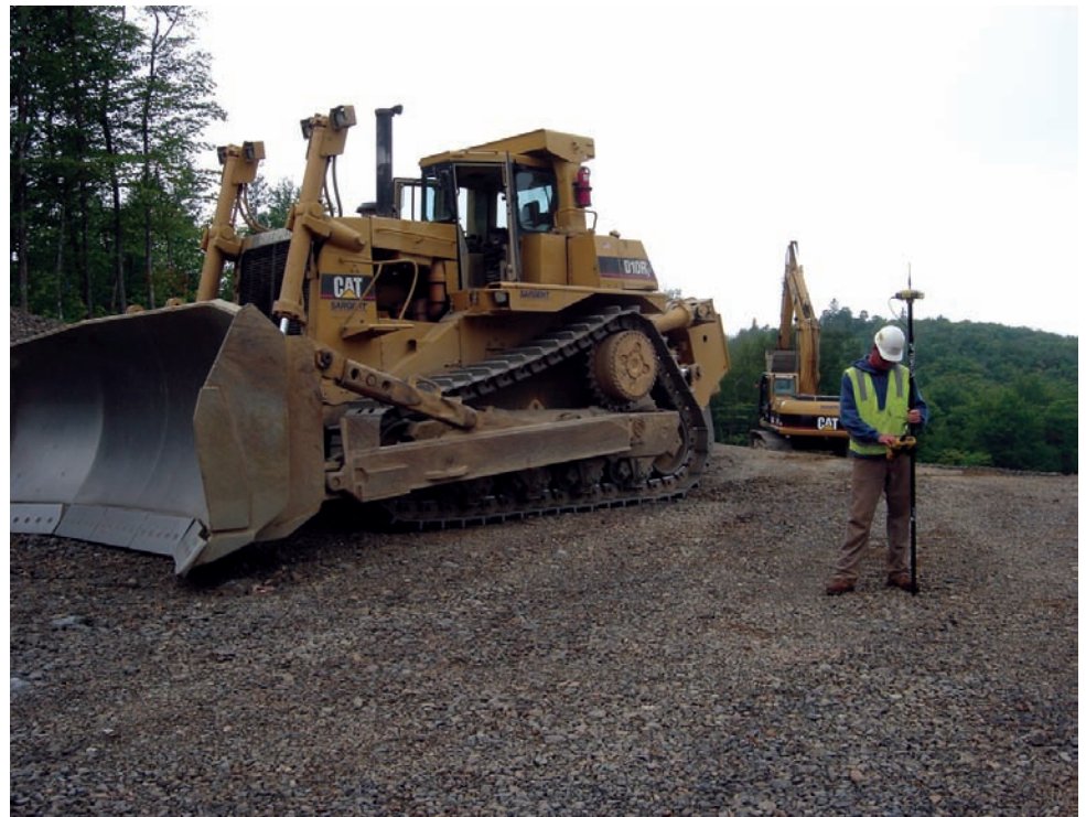
With a Cat D10R equipped with a ripper tooth, at left, a Sargent surveyor uses a second Topcon rover to check road grade.
