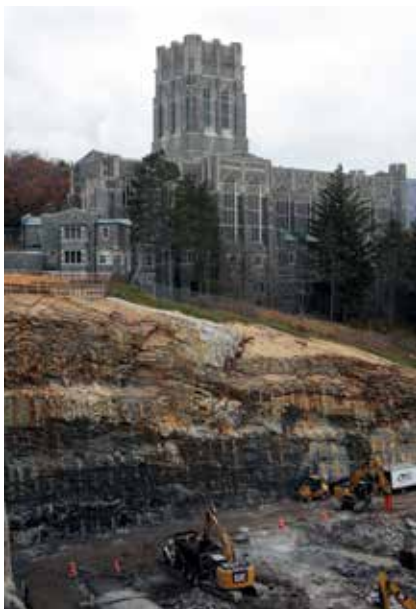
Controlled blasting for 135,000 yds of mass rock and 60,000 sq ft of line drilling/pre-split makes way for the construction of a new Cadet Barracks at West Point Military Academy Campus in New York.
