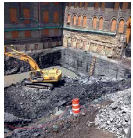
Pictured is the controlled blasting of more than 5,000 cu yds of ledge 20 ft off the existing Goldwin Smith Hall at Cornell University.
