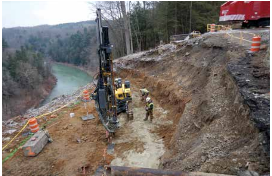
MD&B's West Side Ledger project in Portageville, N.Y., involves blasting a 90-ft rock cut in 6-ft to 15-ft lifts to create a notch for a new bridge abutment. The company will be installing rock dowels the entire way down to support the ledge.
