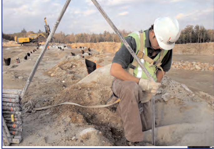
To ensure their accuracy, Pete Marcotte, project engineer for MD&B, employs the Boretrak system.
