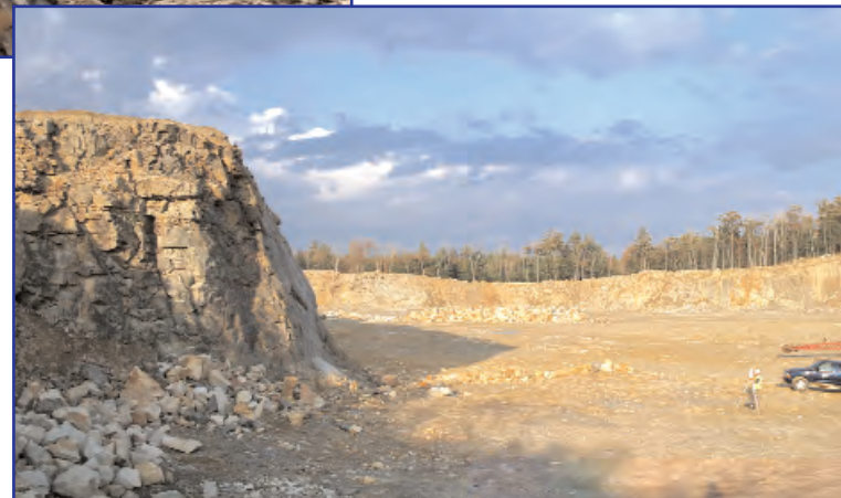
In a nod to the sophistication of the business, laser profiling is employed to ensure the most precise preparation for a blast.
