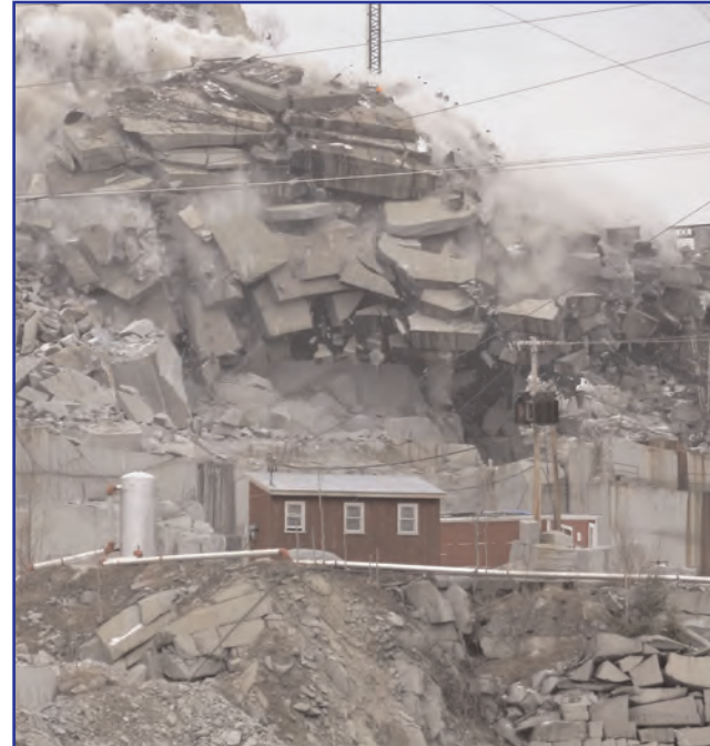
Removing waste rock at Rock of Ages in Barre, VT; MD&B have executed over one million blasts in their 40 years.
