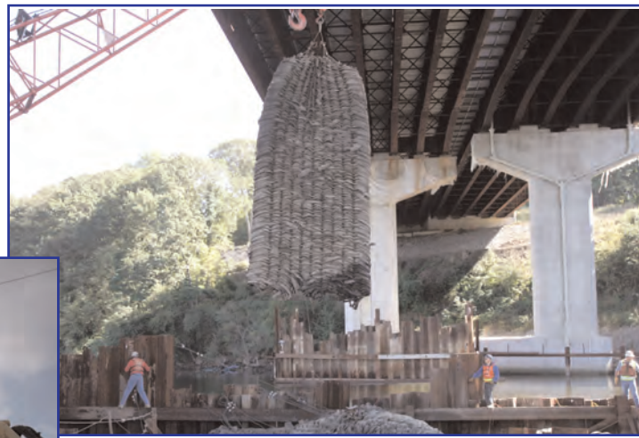
The placement of blasting mats on the Sikorsky Bridge project in Connecticut.
