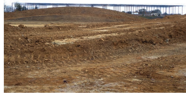
A stockpile of graded material is stored for future use in front of the steel framework of one of the three proposed Lickdale Logistics warehouses.
