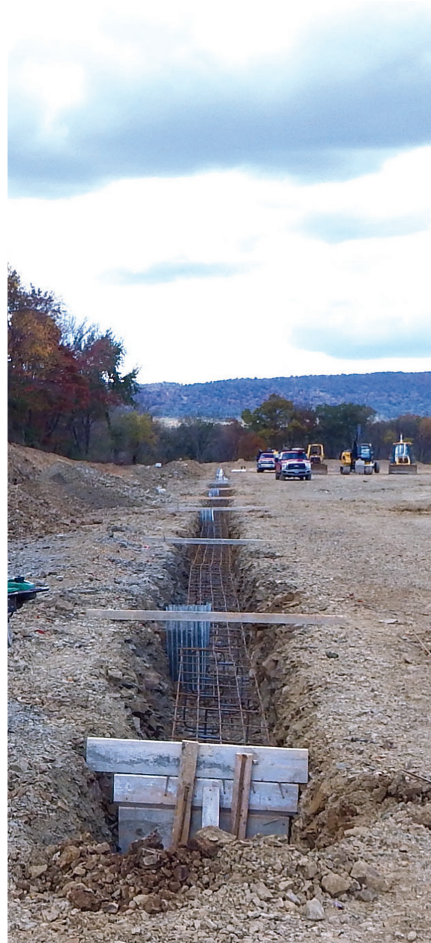
As part of the Lickdale site prep work, MDB blasted 17,000-yards of material. This trench was part of that blasting.
