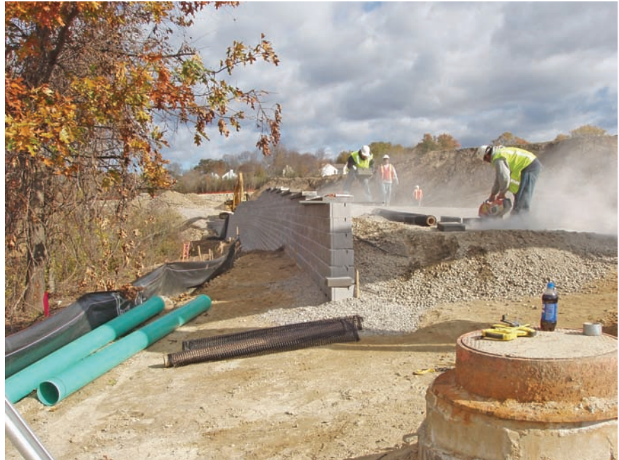
One of six Versa-Lok retaining walls is erected. Walls total 28,000 square feet.
