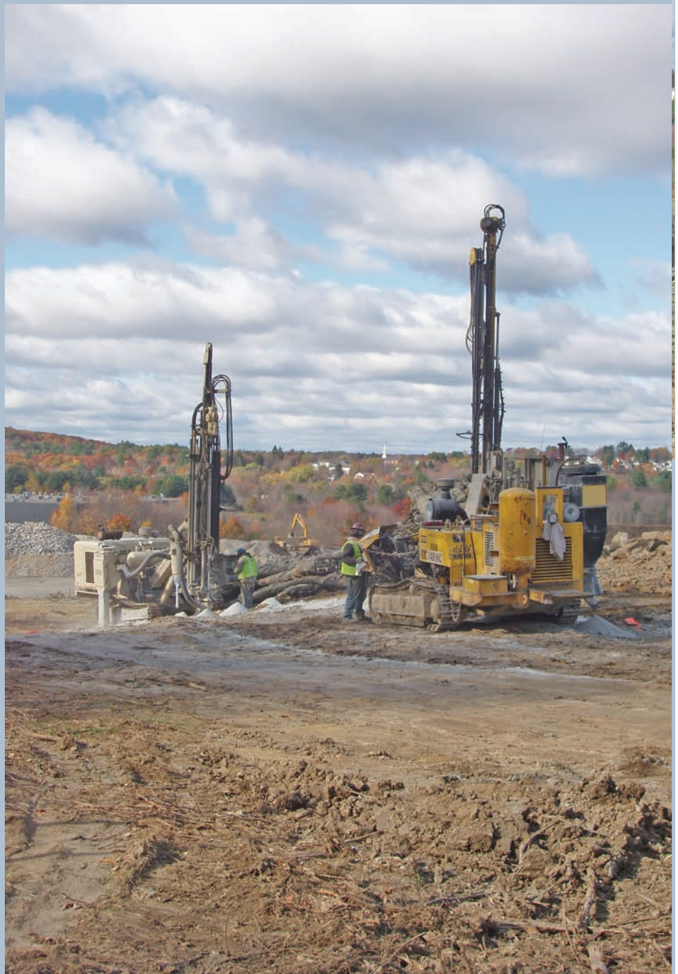
Maine Drilling and Blasting uses Atlas Copco ROC 748 and Ingersoll Rand 590 drills on J. Masterson Construction Corporation's Haverhill Commons job site.
