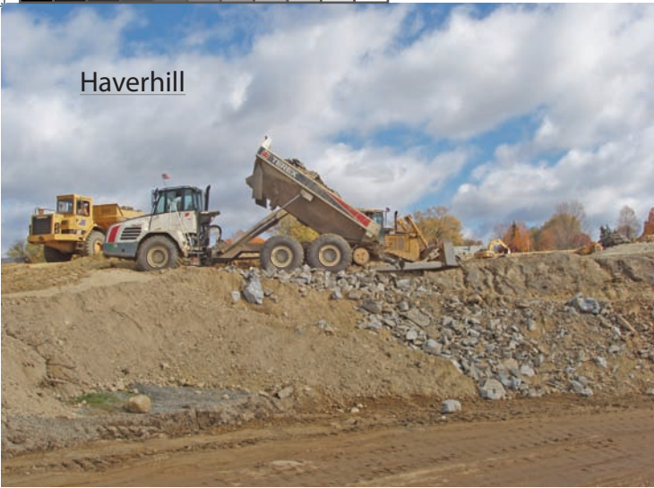
A Terex truck discharges shot rock while a CAT truck passes with another load of rock.
