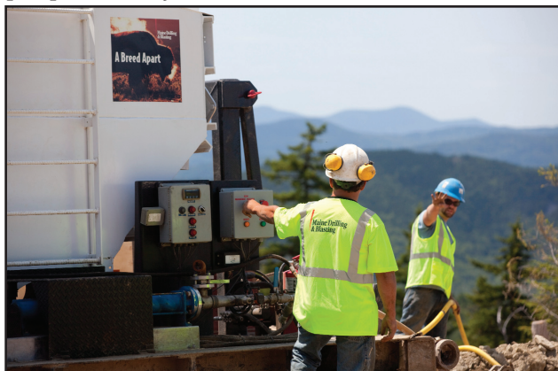
MD&B crew prepares to load holes with the bulk skid pumping unit.
