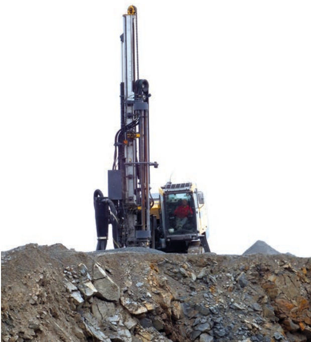
An MDB drill rig operator works atop a bench in a newer area of the pit.
