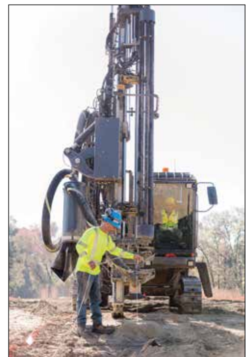
Crews drill a hole using one of five Epiroc T40 Drill Rigs added to the Precision Blasting fleet in 2023. (Photo courtesy of Precision Blasting)
