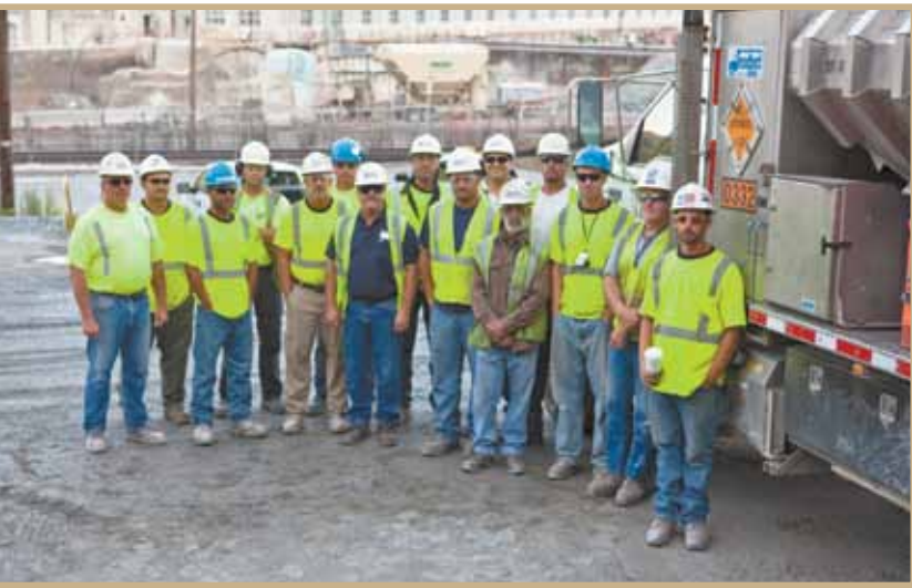
It takes a special breed of individuals to maintain the quality drilling, blasting and rock bolting work being performed at the Holtwood Hydroelectric Project.
