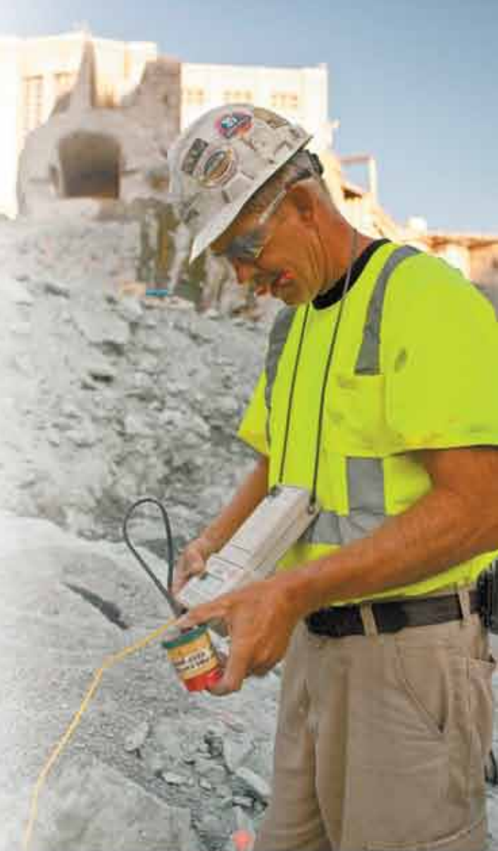
Blasting superintendent, Dana Lawrence, communicates with each detonator via a handheld computer to ensure proper timing for each blast round.
