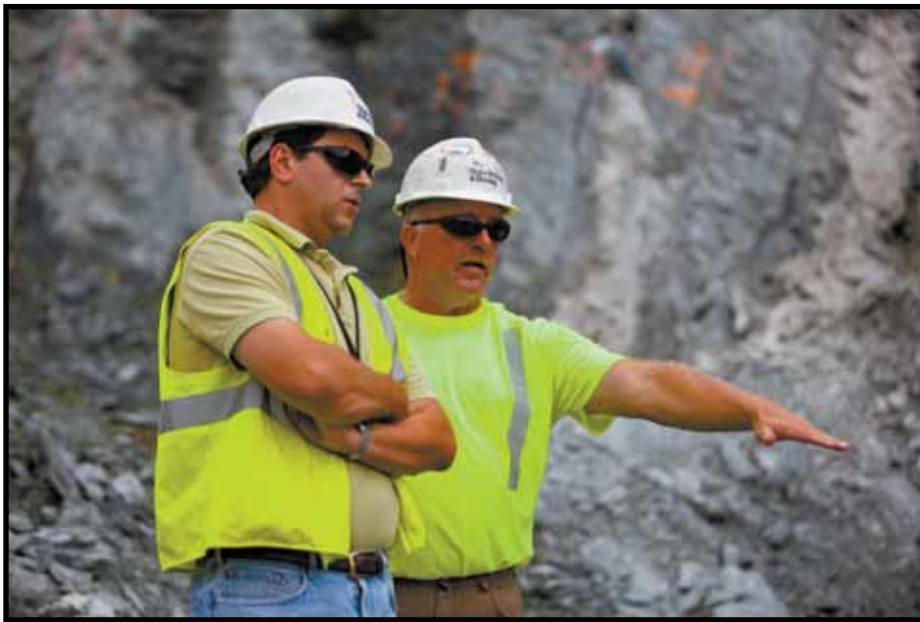
Safety director Rick Galletta and project superintendent Hod Wing reviewing the hazards of the congested work site. The construction team proactively approaches the future hazards working in the New Powerhouse excavation.
