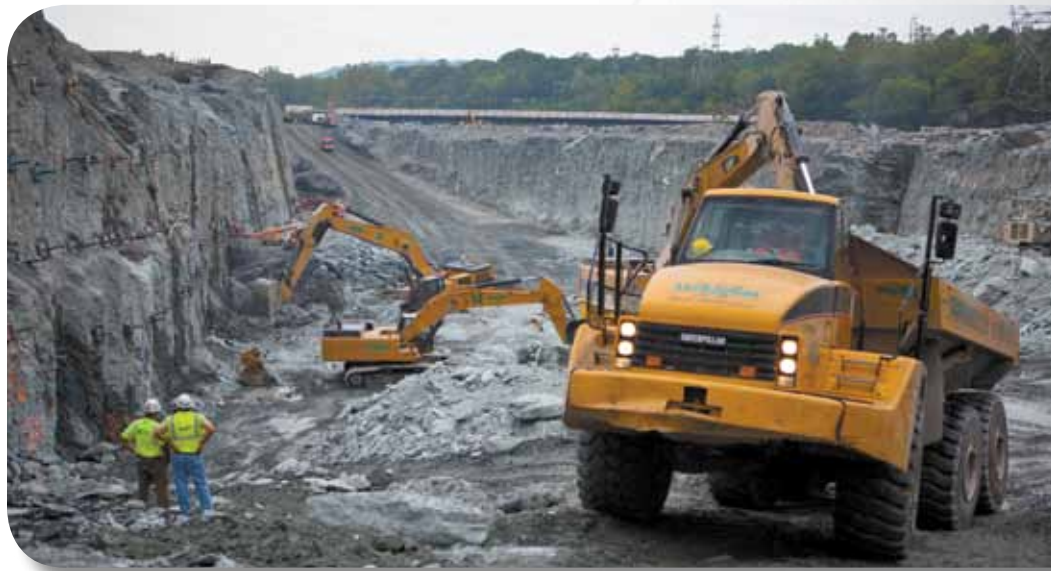
A congested work site requires each individual to keep an eye out for each other.
