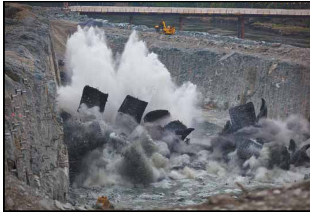
The view from a safe distance of one of the many production blasts. Shown here is a blast yielding 3,000 cubic yds.
