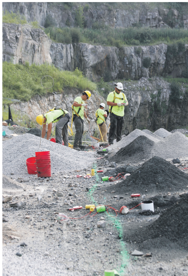
The blast crew at work. Blasters Jason Guilmette and Blake Kerrigan (white hardhats) begin the process of loading explosives, while laborers Owen Gannon and Nathan Heroux (yellow hardhats) get stemming ready for confinement of holes once they are loaded.
